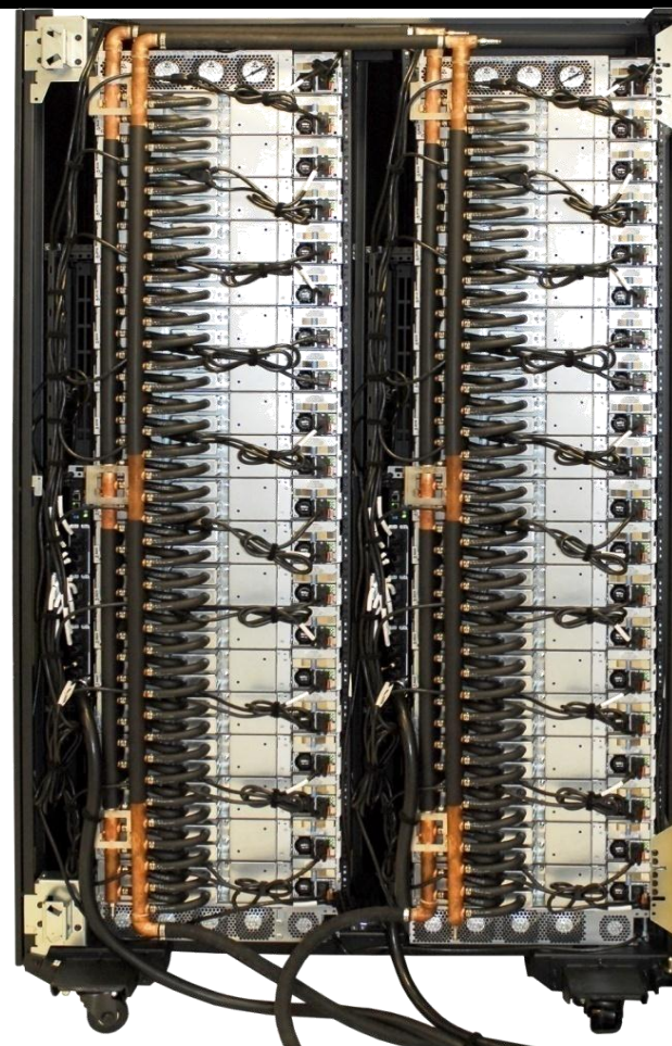
iDataplex DWC Rack w/ water cooled nodes (rear view of water manifolds)
